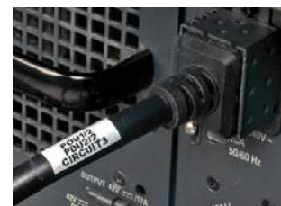
Electrical Infrastructure Labeling
