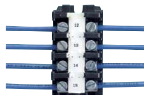
Terminal Block Labeling
