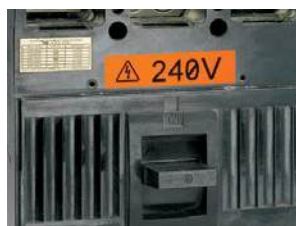
Electrical Hazard Labels
